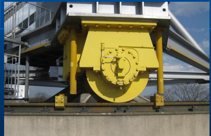
Ibaraki station damages
